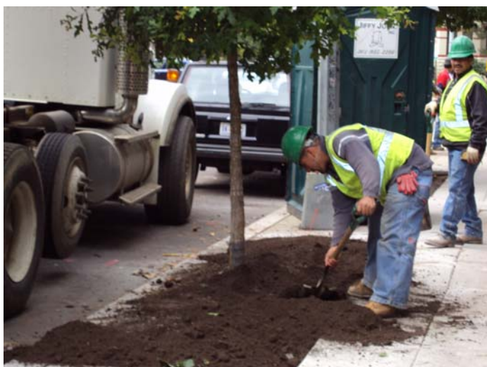
Workers spread topsoil in an expanded tree-box on the 1800 block of Kalorama Road. Photo: Steve Mckindley-Ward
